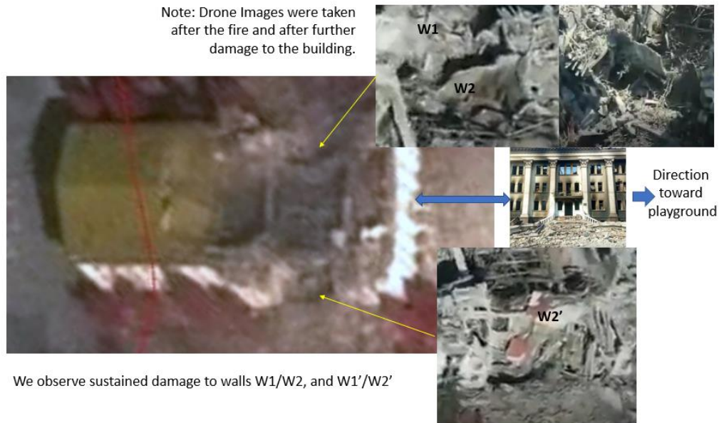
Figure 2: We analyze in this report the damage to the various walls to determine the size of the explosion that is consistent with the damage observed from the satellite image. However, we also use some of the screen capture from the subsequent drone videos but only to substantiate what we see not to estimate the damage since we don't know if the damage in the insets are due to subsequent explosion, fire etc. [Source: https://twitter.com/Militarylandnet/status/1509438591952424962?s=20&t=mmNFdiM4gpjV-LLotC8CrQ ]
